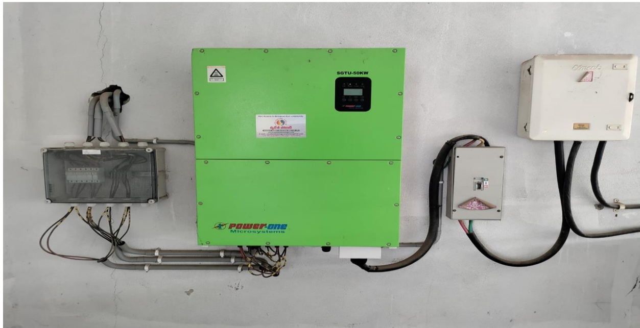
Wheeling to GRID connection
