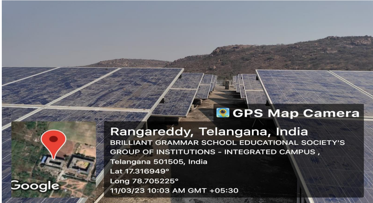
View of Solar Power plant 75 KWp.
